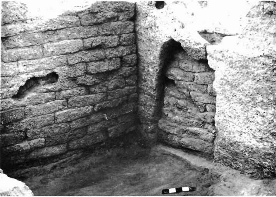
Plate 12. View of the arched passageway from the ceremonial rooms to the service quarter. Here, the door is viewed from the temple courtyard, still sealed by the brick packing. The north arrow points to the tablet mentioned as bearing the name Ninkarrak.
